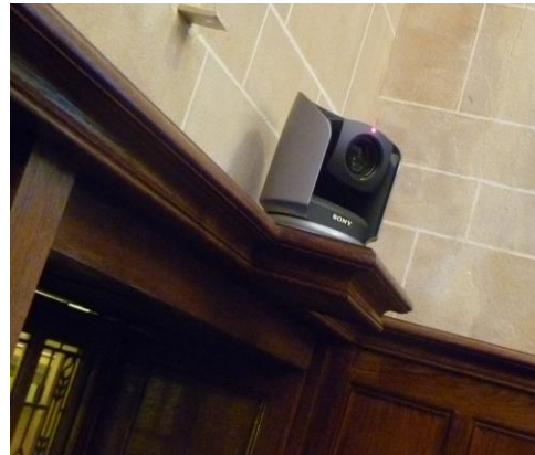
One of the wall-mounted court cameras
